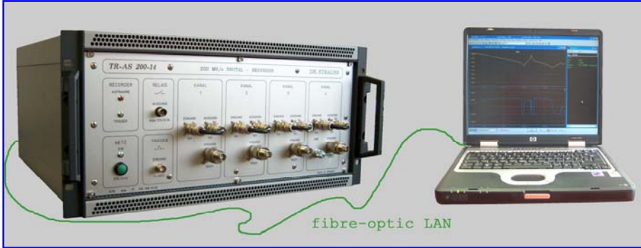
TR-AS® RC with 1 to 4 measuring channels located closed to the test field
